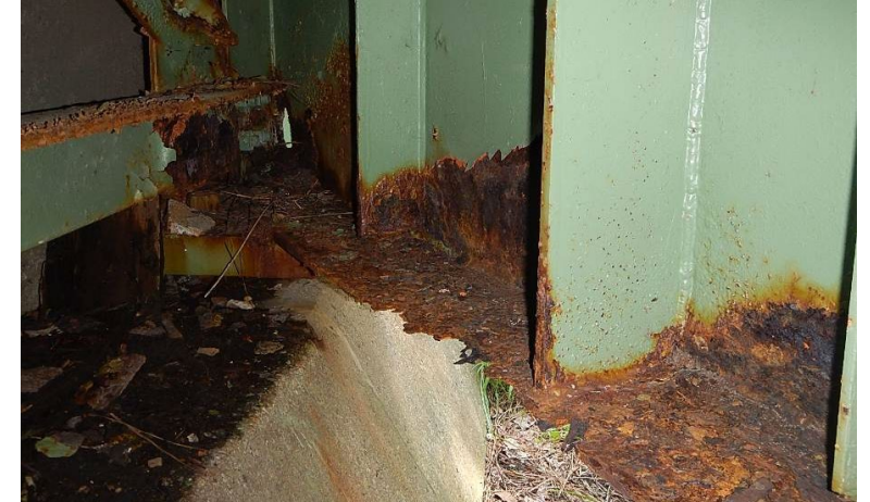
Poor (Structurally Deficient)
